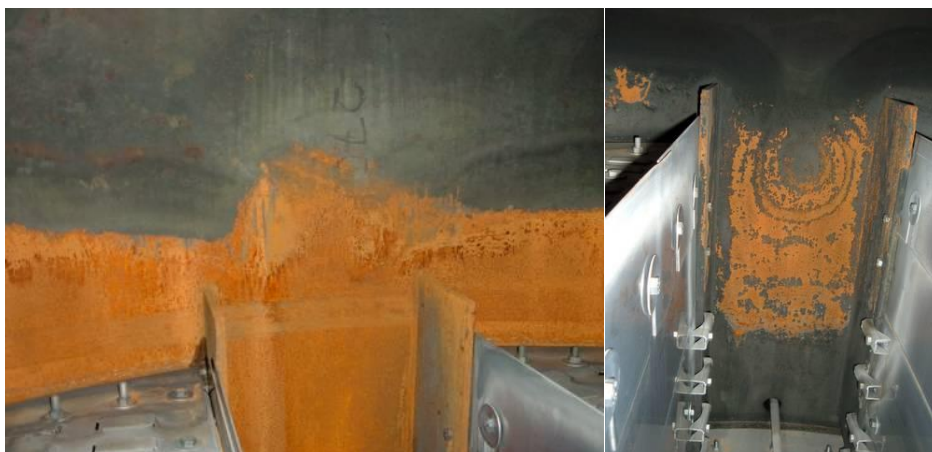
Figure 8. Contactor Wall Corrosion in Tray Liquid holdup Area and Downcomer
