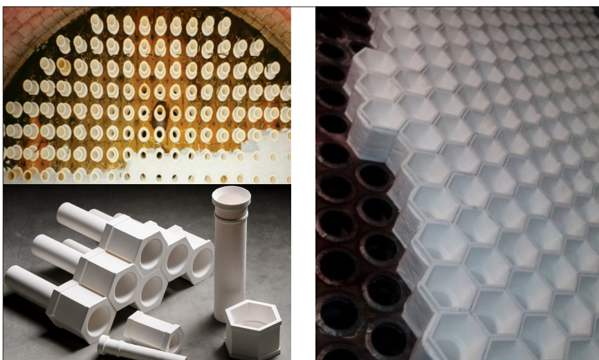
Figure 3 Types of ceramic ferrules, installed view: (a) Conventional ferrules before final refractory installation; (b) Hex-head ferrules (courtesy of Blasch Precision Ceramics)
