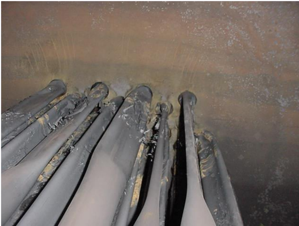
Image 1. Failure in the Waste Heat Boiler due to overheated tubes
